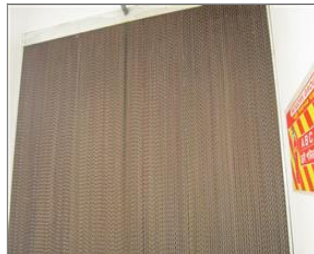
Photo of the inside of the main production hall Air cooling system.JPG
