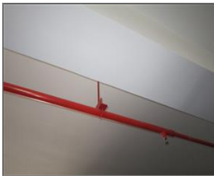
Photo of fire safety equipment Sprinkler.JPG
