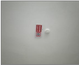
Photo of fire safety equipment Smoke detector.JPG
