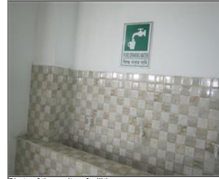
Photo of the sanitary facilities Drinking water facility.JPG
