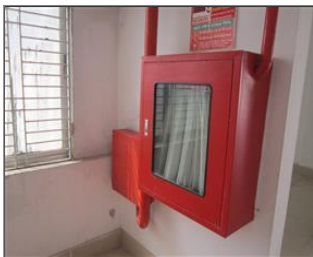
Photo of fire safety equipment Water hose reel.JPG
