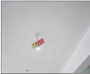
Photo of fire safety equipment Emergency light.JPG
