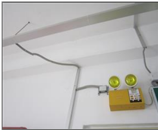
Photo of fire safety equipment Fog light.JPG
