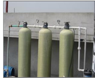
Photo of the sanitary facilities Drinking water filtering system.JPG
