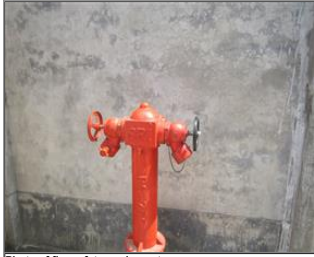
Photo of fire safety equipment Fire hydrant point.JPG
