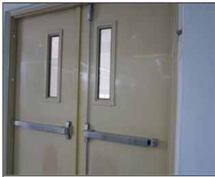
Photo of fire safety equipment Fire rated door.JPG
