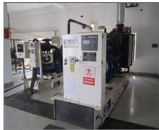
Photo of the inside of the main production hall Generator.JPG
