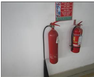
Photo of fire safety equipment Fire extinguishers.JPG
